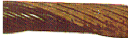
Figure 23: Corrosion in the second and third layer of the rope
