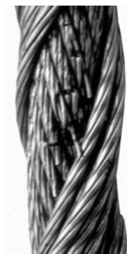
Figure 4: Broken wires in second layer of strands
