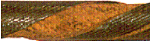
Figure 22: Corrosion in the first and second layer of the rope
